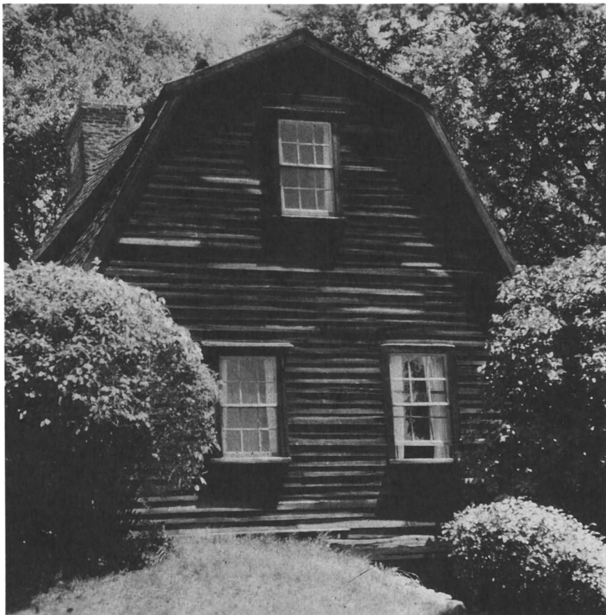
Figure 1. Old Fairbanks house at Dedham, MA, built in 1637. Most of the white pine clapboard siding was replaced in 1903, and it has withstood 85 years without paint.
